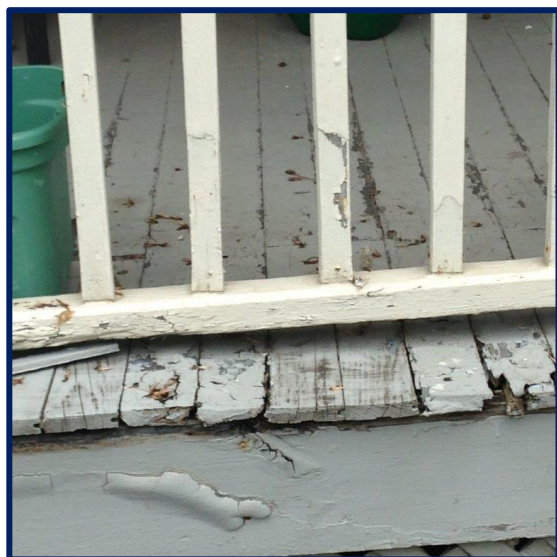
Image 9 Railing and porch with lead paint
