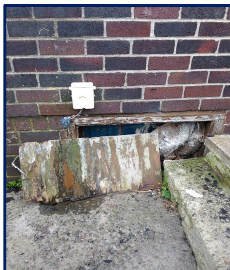
Image 10 Old boarded window with lead
