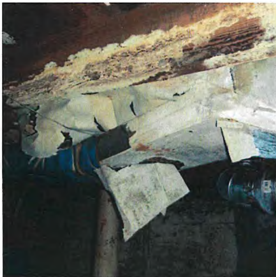
Basement view showing significantly damaged ACM and compromised floor joists.
